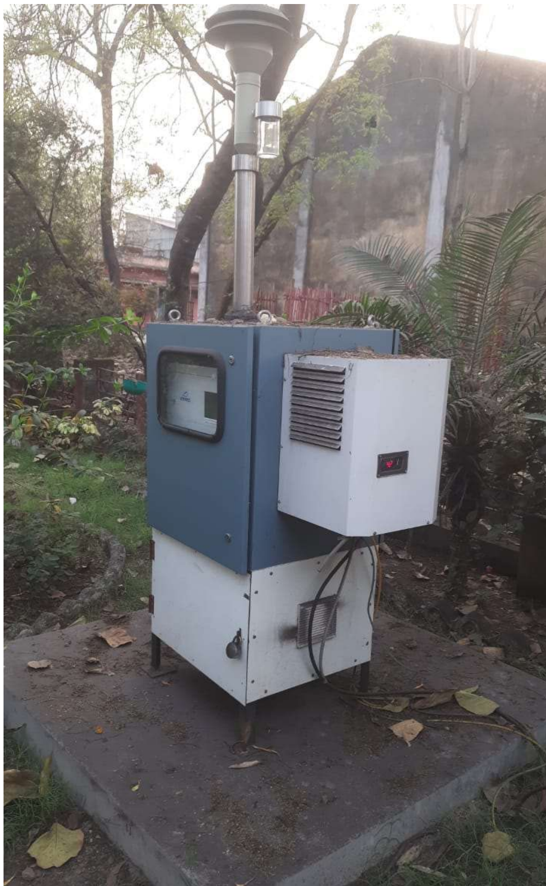
Picture 14 – PM10 Analyser Installed
