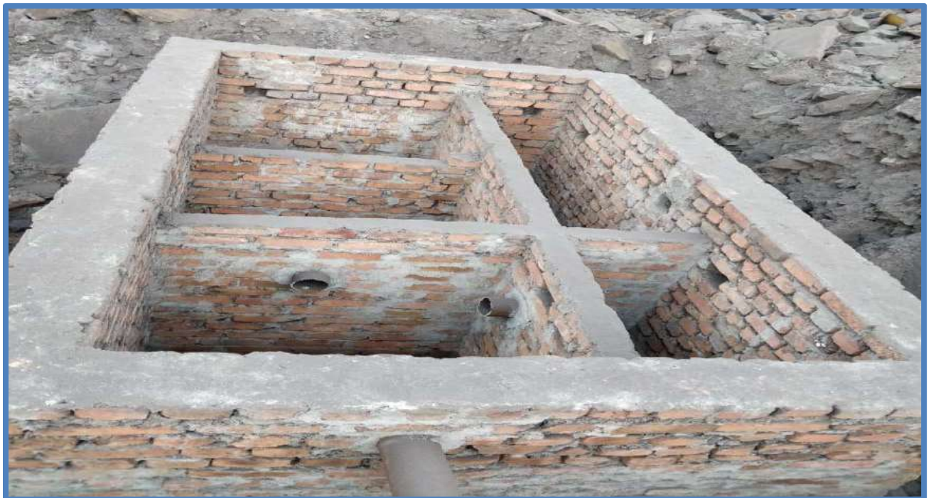
Picture 10 – Oil & Grease Trap
